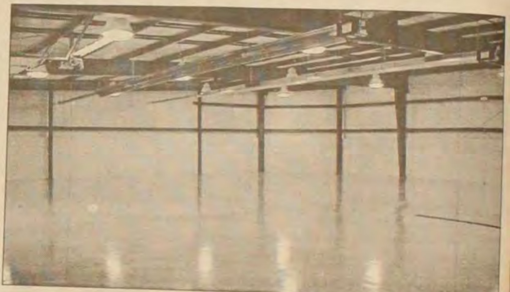
The floor of the 5,000 square-foot storage addition in Templeton Hall was painted and sealed this week. Logos will also be added to the floor.
