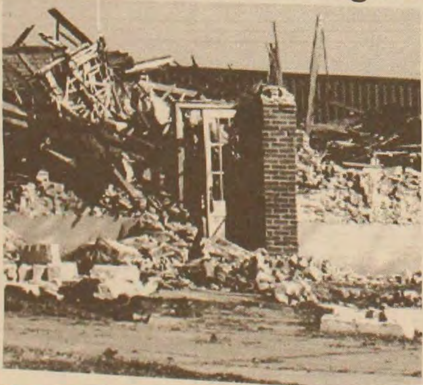
The building which once housed the art department is now a pile of rubble. Students and faculty salvaged old pottery and paintings before the destruction began on Monday, Feb. 6.
