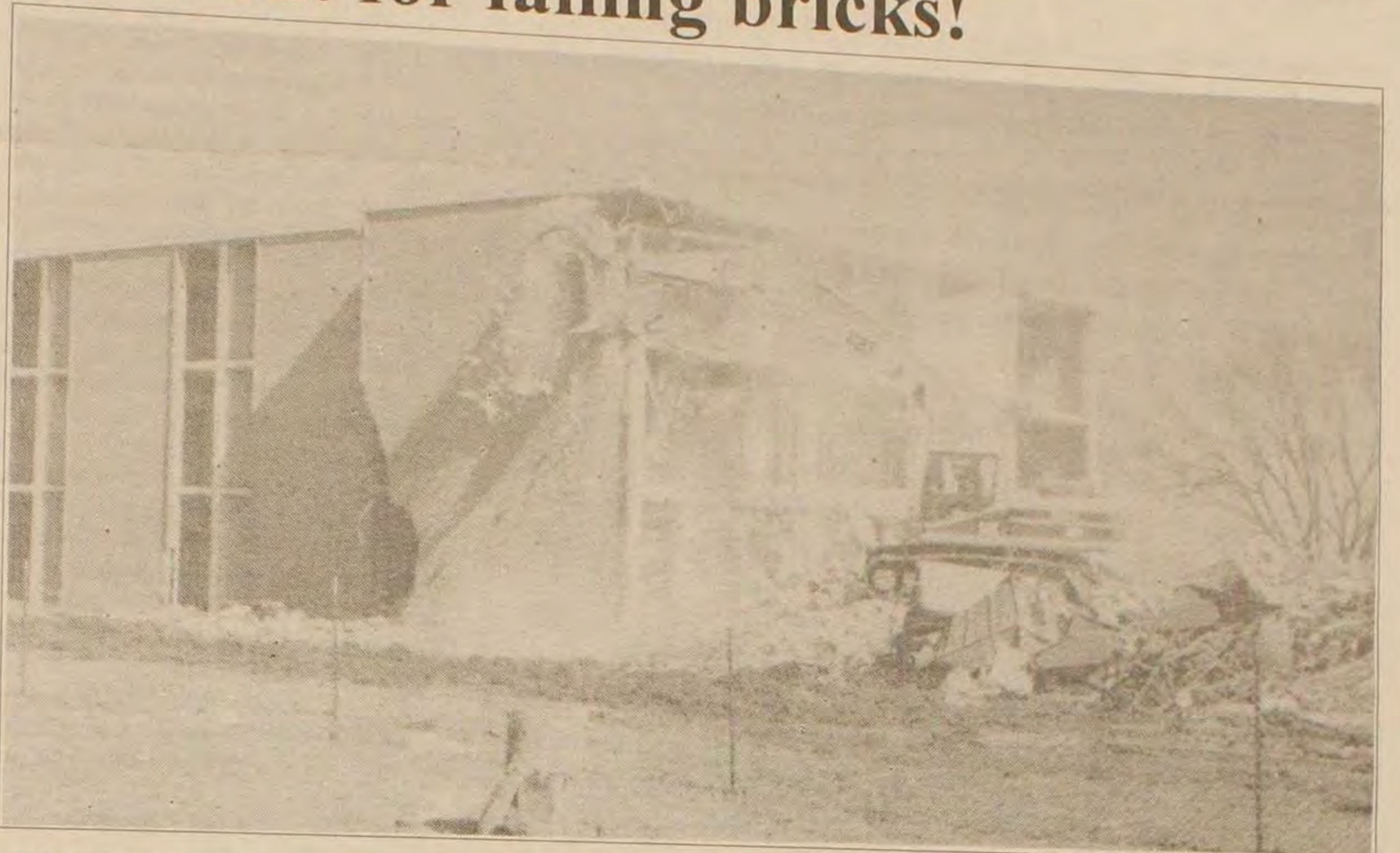
Even though a bulldozer is not quite as impressive as a wrecking ball, the effect is similar. Demolition of Bittinger Hall began this week and will soon be completed.
