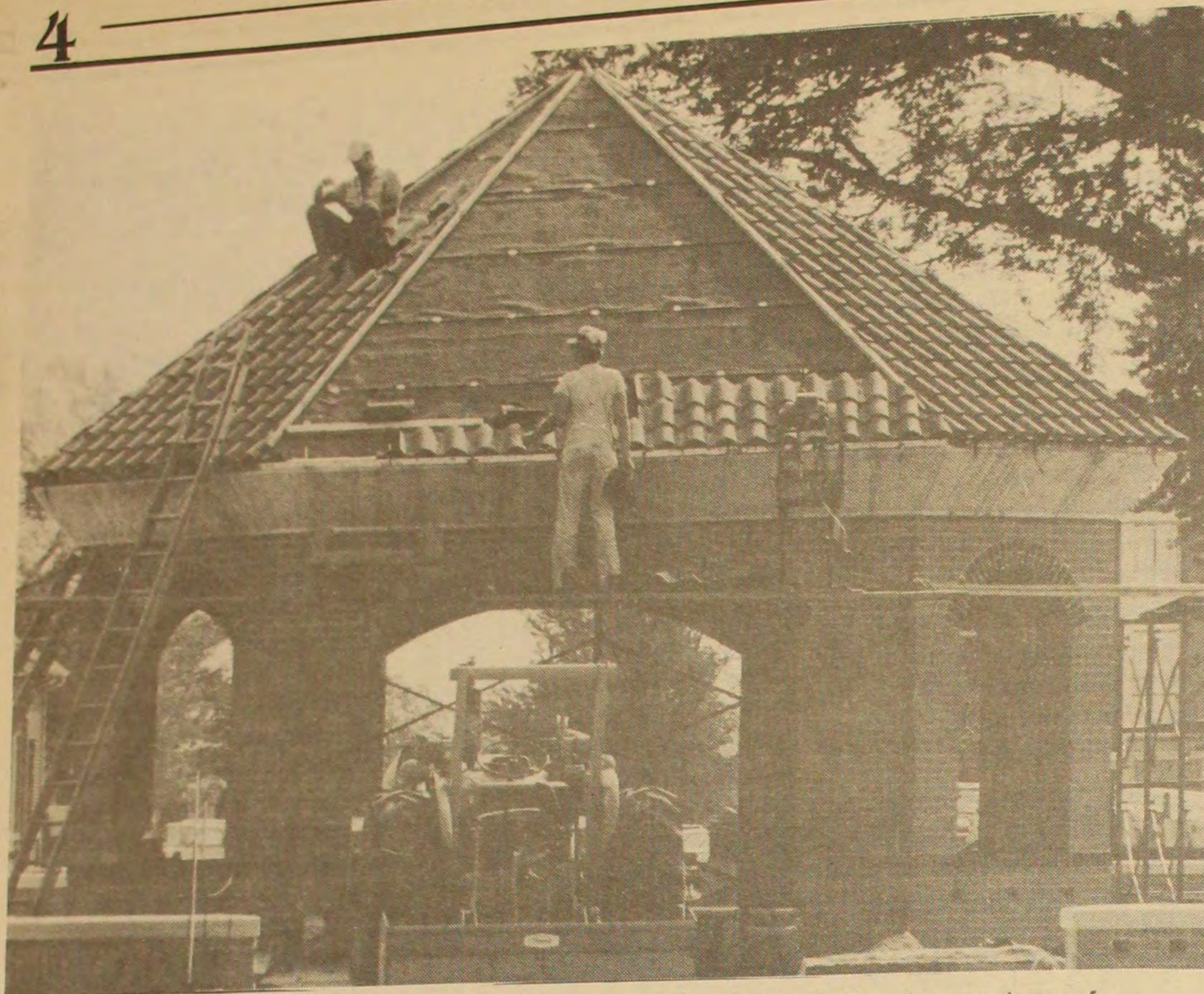
Local carpenters take advantage of the warm weather to finish tiling the gazebo roof. Jack Patiño/Spectator
