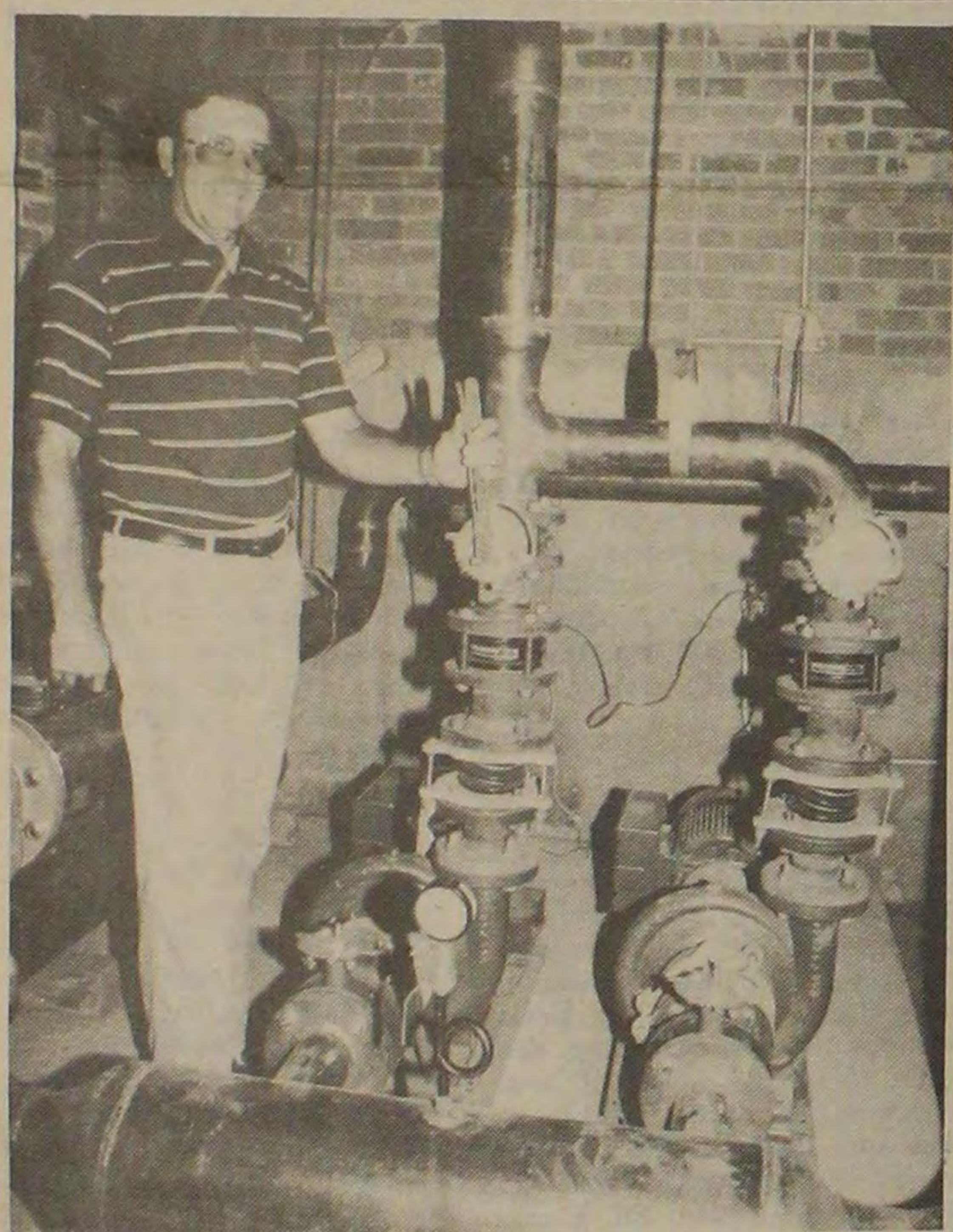
Merrin Godfrey and the Dotzour heating system
