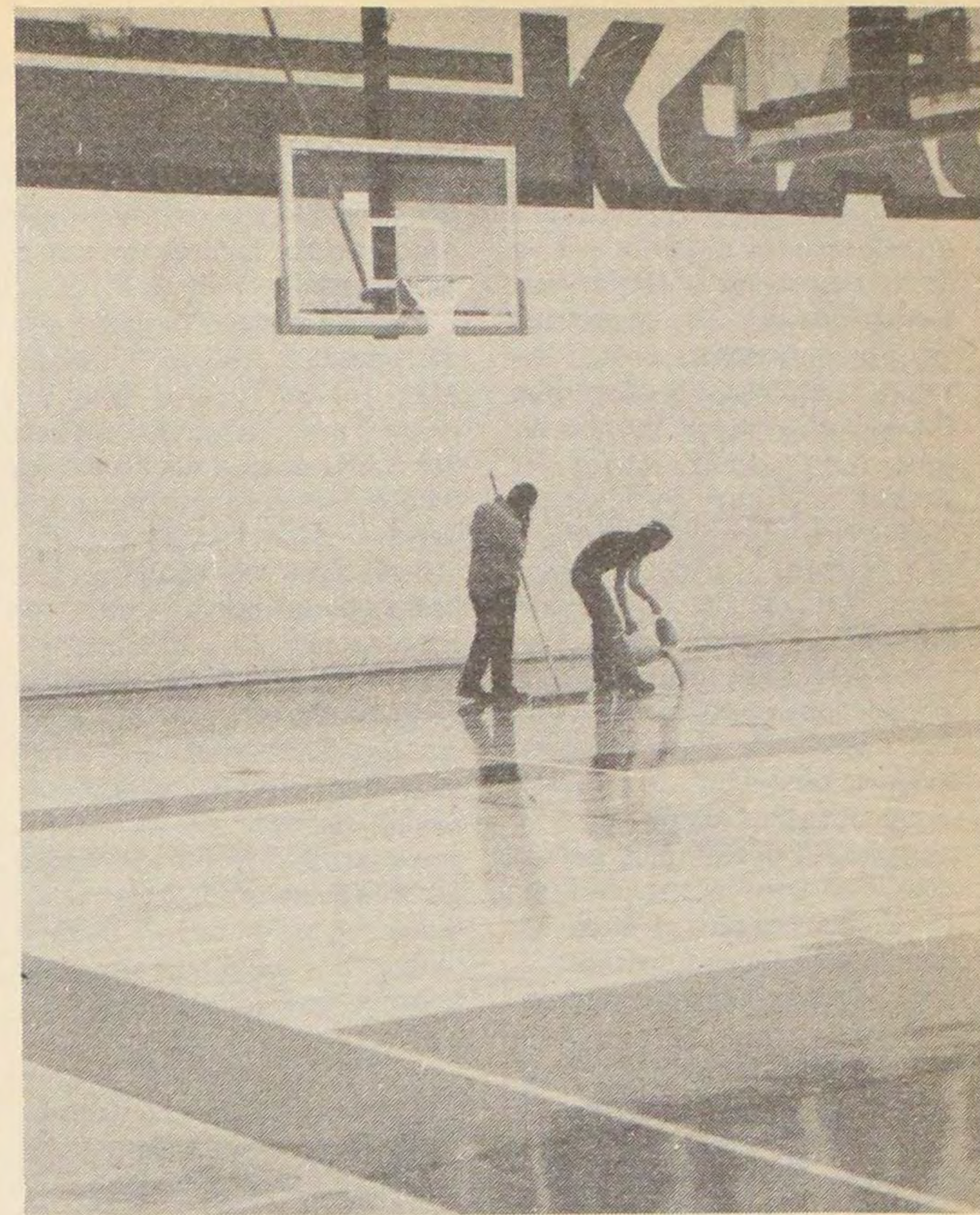
Workers "pour the track" in the new Sports Complex. Absolutely final completion has been set for early January. We're not holding our breath.
